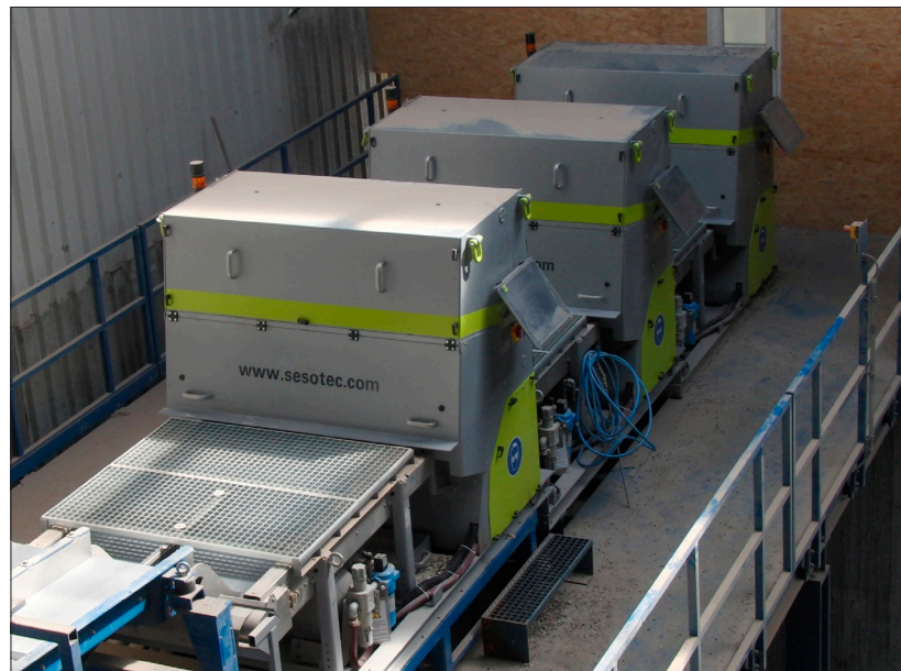
Fine line at the Reiling glass recycling plant with three Sesotec K9 systems.
